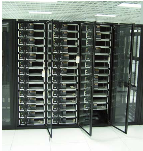
Over 200 SNV-12 Signal-and-Noise Voters are installed in China's air control centers. Pictured are some of several racks of the SNV-12s in Guangzhou.
