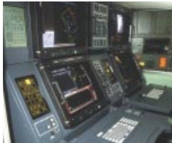
Fire Distribution Center
