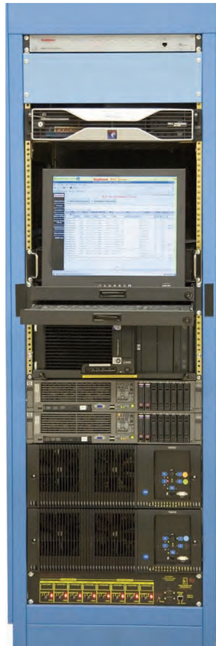
Photo Caption: Raytheon's P25net Solution rack installation
